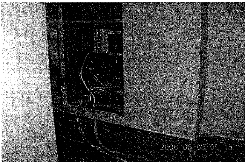
Licensed Medicinal Marihuana Grow- Electrical Safety Hazard Work performed without permit or inspection.
