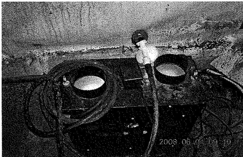
Licensed Medicinal Marihuana Grow- mould and electrical safety issues.
