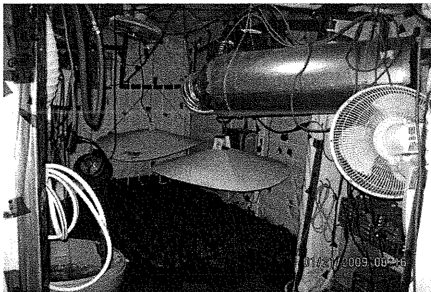
Licensed Medicinal Marihuana Grow- Various electrical and fire safety issues.
