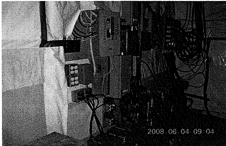
Unapproved electrical distribution with non CSA equipment. 110 volt receptacles used with 240 volt equipment. Electrical equipment suggests a very large quantity of plants, considering one ballast per light and one light handling from 12-16 plants
